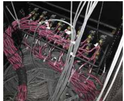
A look at some of the cabling infrastructure implemented in the upgrade project.
